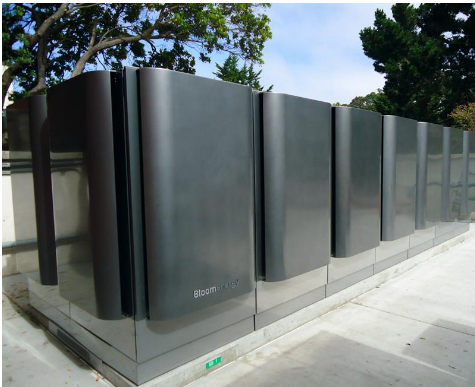
Figure 1.3: Bloom Energy Server powered by SOFCs. 18
