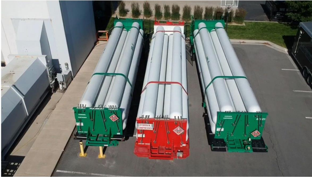
Figure 1.4: The hydrogen fuel cells used by Microsoft as backup generators for data center servers. 19
