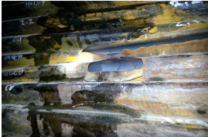
Figure A.1: Failed tubes on division wall of Unit 2 boiler from station A.
