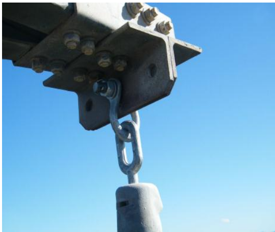
Figure F.3 Installed OHL fitting
