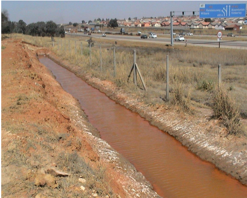
Figure 1: Impact of low pH on the trench.
