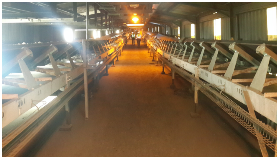
Figure 1.2: Typical Conveyor within the Port of Richards Bay (PORB)
