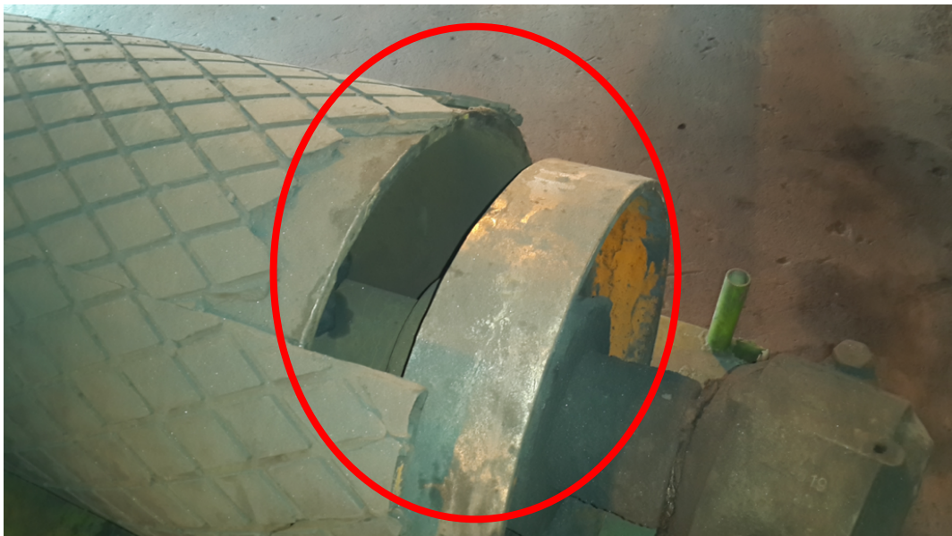
Figure 4.5: Pulley end disk failure
