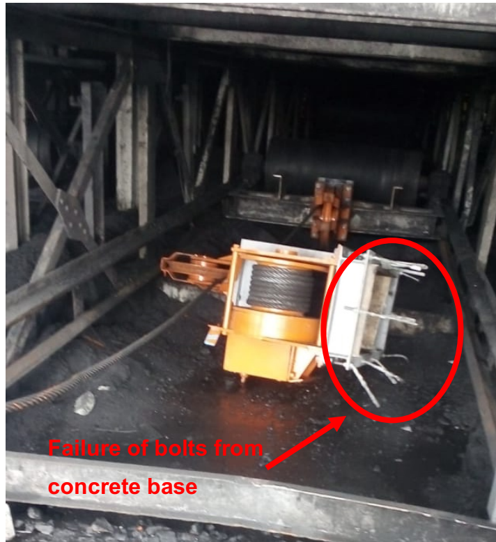
Figure 4.11: Take-up winch failure
