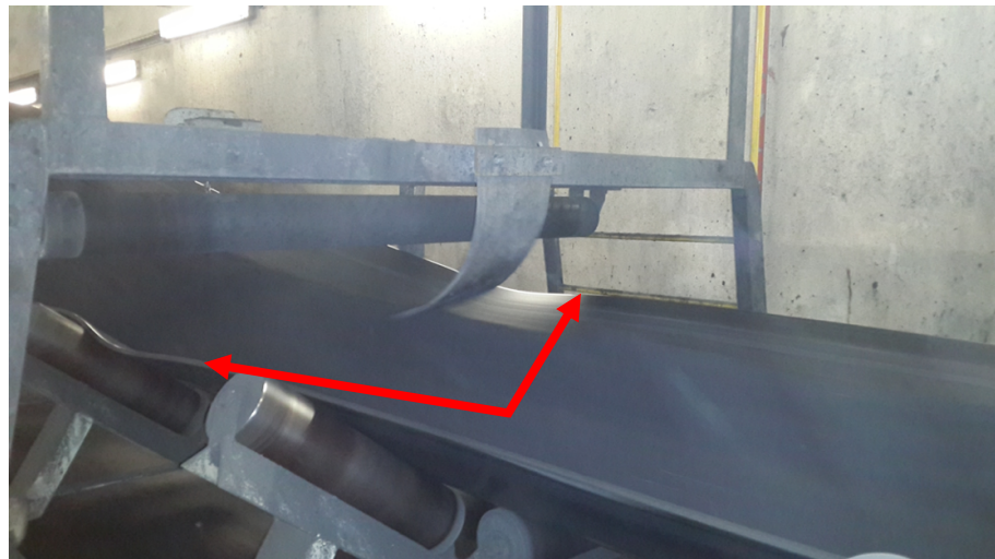
Figure 4.9: Belt edge buckling under load
