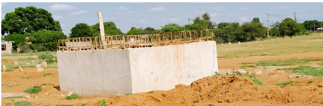
Figure 14:A utility hole which is part of the water project along the Pavement, Vuma road.
