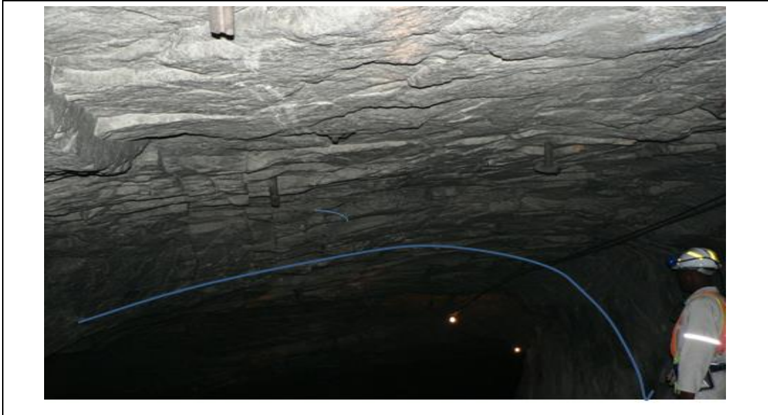
Figure 2.1.8_1 Induced fracturing in the hanging wall of the Merensky Reef
