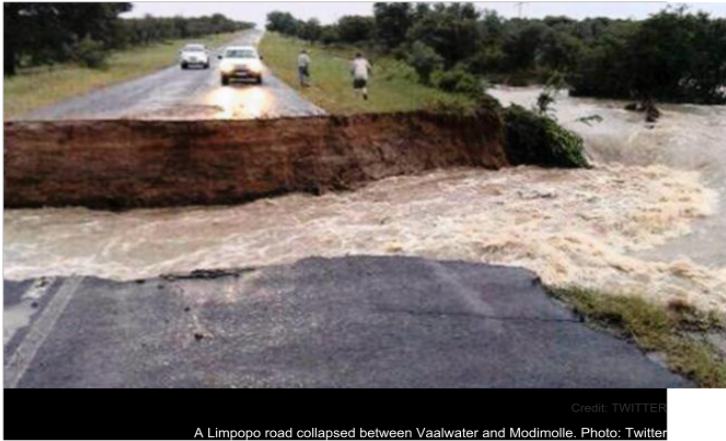
A Limpopo road collapsed between Vaalwater and Modimolle. Photo: Twitter
