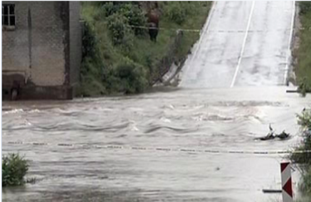
Police say a dam wall in Bela Bela collapsed under pressure due to heavy rainfall. (SABC)
