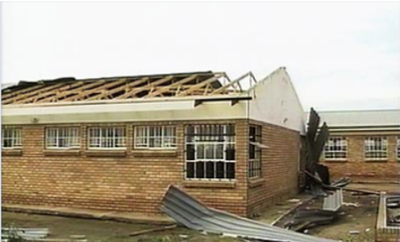
Houses, schools, church buildings, and power lines are some of the infrastructures damaged during the storm. (SABC)
