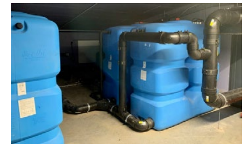
Figure 141 : Rainwater stored and collected under recycling platform used for cleaning and flushing toilets, (Modulo,2019).
