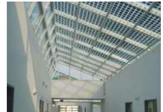
fig. 133. Building Integrated Photovoltaic panel used in skylight design (Unknown, n.d)
