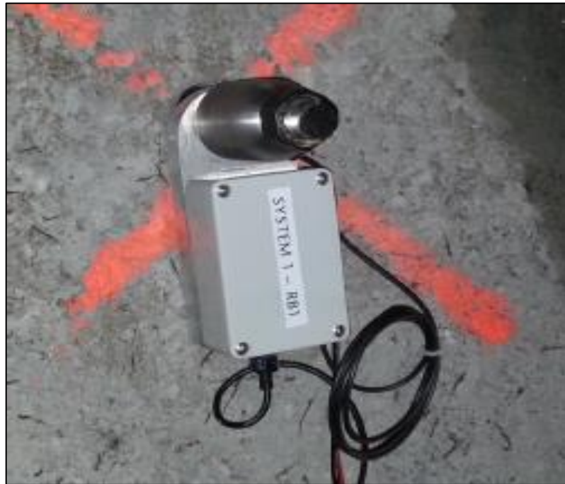
Figure 3.6-3. A smart rock bolt installation in a mine (Eliasson et al., 2014).
