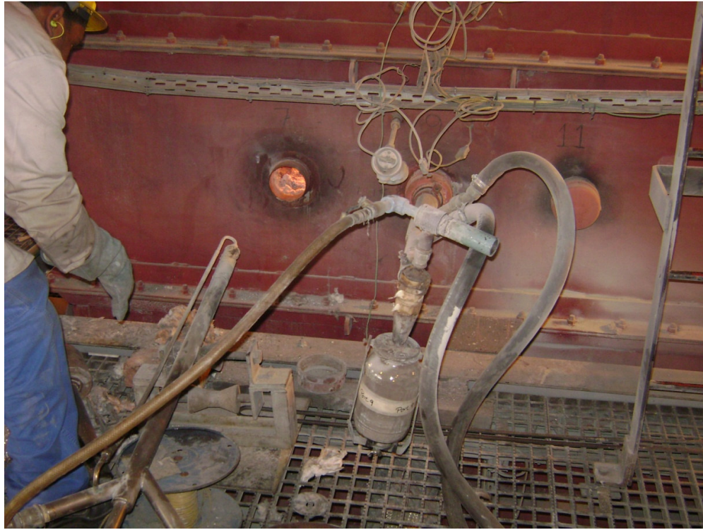
Figure 4.9 Fly ash sampling at port 9 and slagging probe on the floor. The Slagging probe was used to take slag samples which were sent to Van Alphen Consultancy for detailed analysis.
