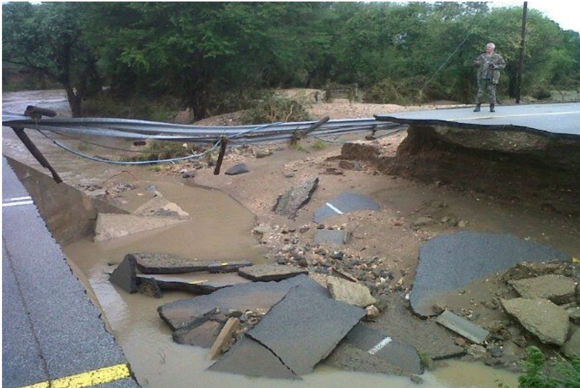
Picture 1: Bridge washed away by floods (Source: Limpopo Provincial Roads, 2012)
