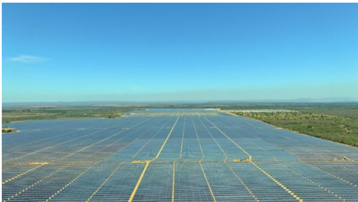
Figure 3.1 - The NDB co-financed solar power plants in Pirapora, Minas Gerais
