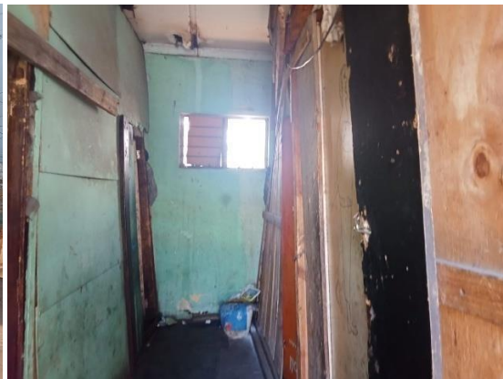
Figure 10: Partitioning using fire hazardous materials
