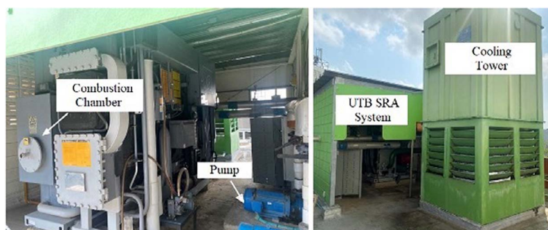
Figure 17. UTB Auditorium absorption cooling system.
