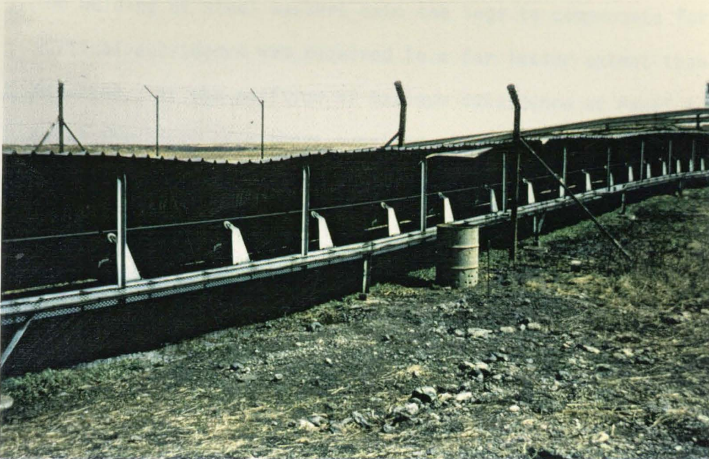
PLATE 10 Compressive strain caused the buckling of the cover plates shown in the photograph.
