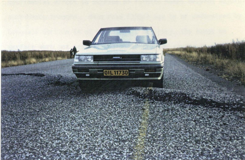
PLATE 3 A compressive ridge which formed on an unused section of a tarred road.
