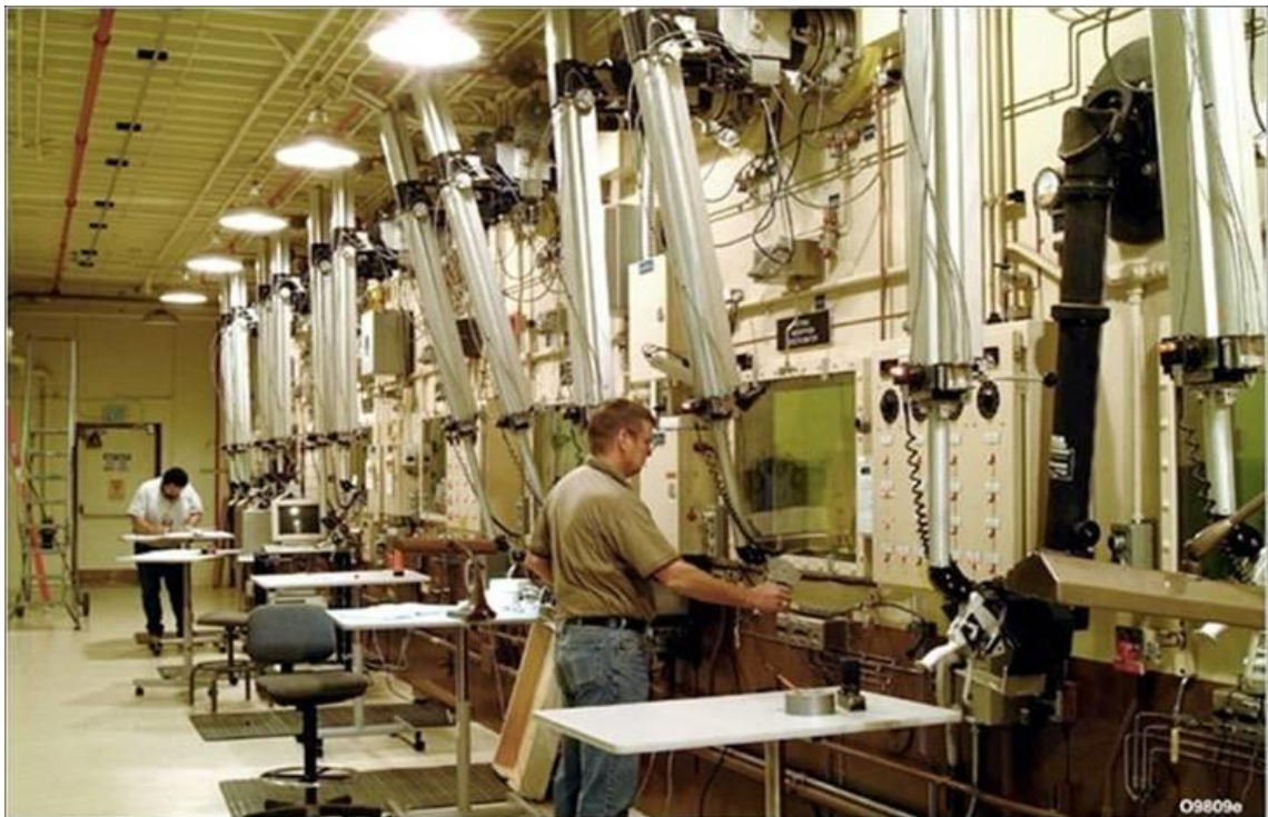
Figure 1.1: Highly shielded hot cells for extremely high activities (source: https://inlportal.inl.gov/portal/server.pt/community/materials_characterization/698/hot_cells/8075 ).
