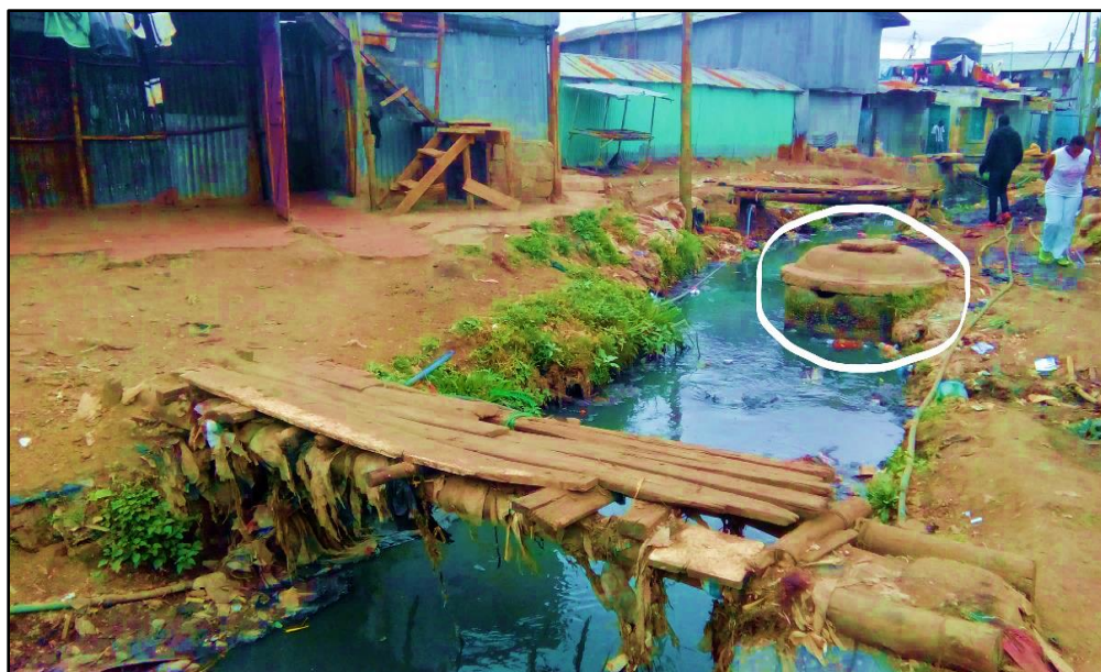
Figure 4.16: The open wastewater disposal drain in Zone 48 (see formal sewage manhole – circled, but no connection for the settlement)
