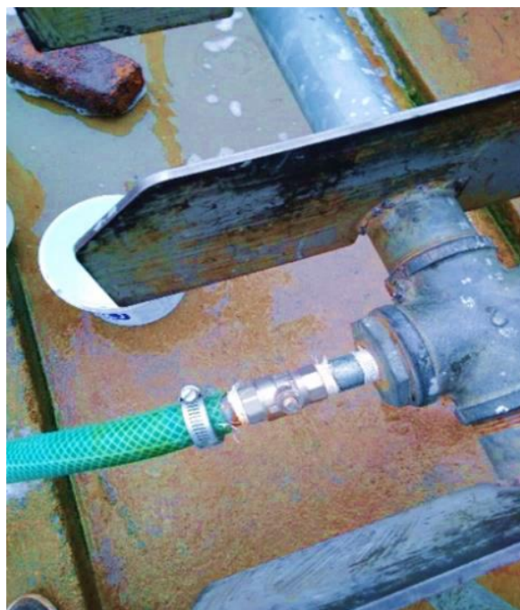
Figure 6.8: Illegal connection to a household in Section D
