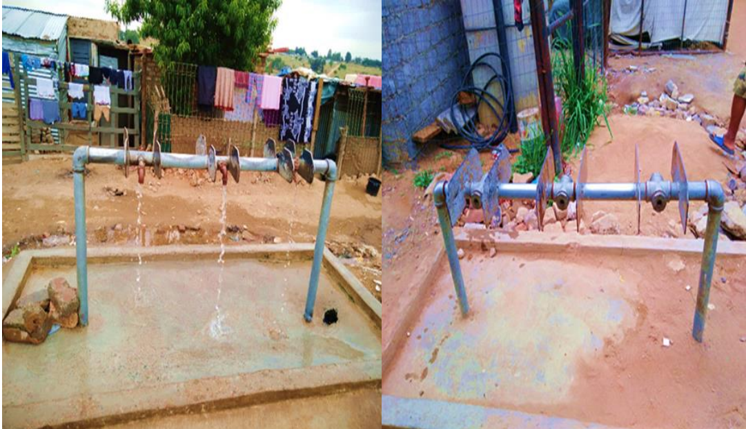
Figure 6.6: On the left, leaking taps at a standpipe and on the right, "an all taps" closed standpipe
