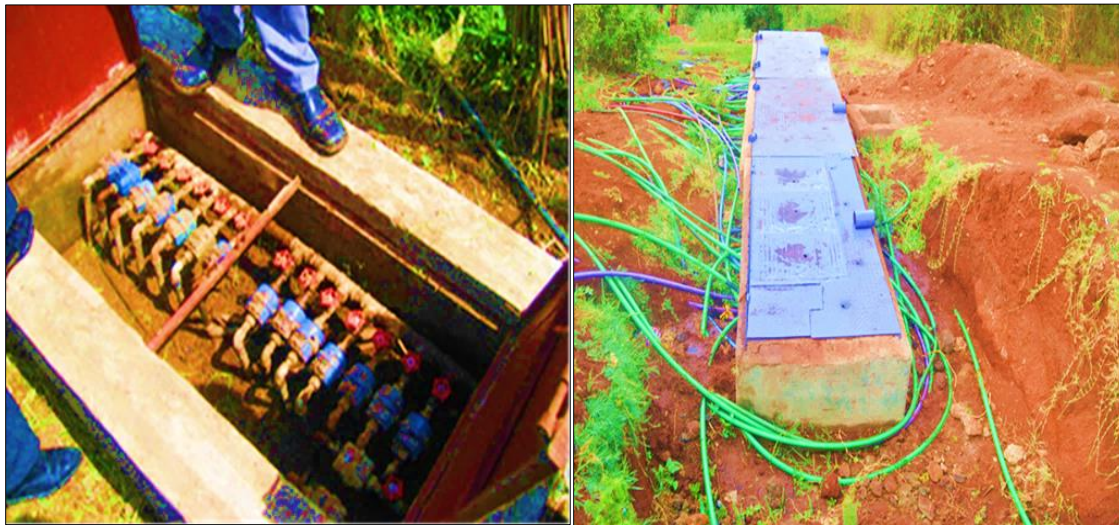
Figure 4.7: On the left, the view inside a chamber. (Source: KFTS, 2008). On the right, pipe connections from the chamber. (Source: NWSC, 2019).
