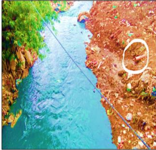
Figure 4.14: An effluent pipe (circled) emptying wastewater into the Ngong River in Sisal Village
