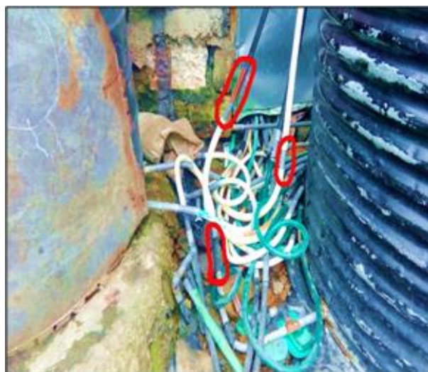
Figure 5.4: Color coded pipes at water tanks by vendors (circled in red)
