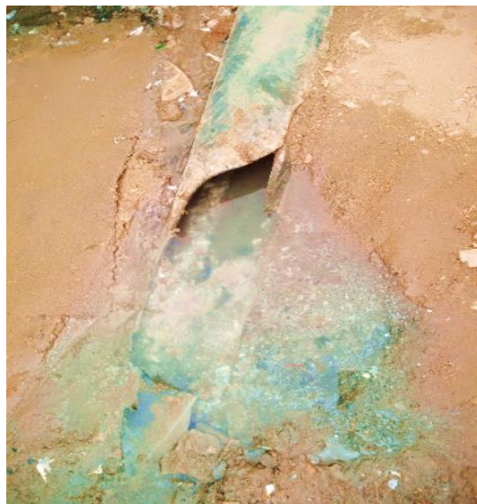
Figure 6.18: A burst wastewater pipe in Section B
