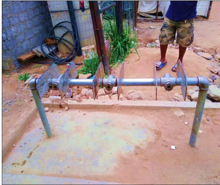
Figure 7.1: A disconnected standpipe in Section D
