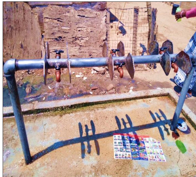
Figure 6.5: A standard standpipe in Section D with six taps
