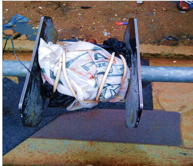
Figure 7.2: Improvised repairs of a leaking tap by residents in Section E
