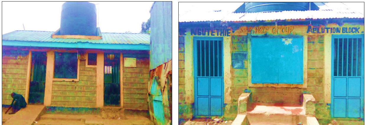
Figure 5.5: Dysfunctional donor funded ablution blocks operated by CBO and SHG
