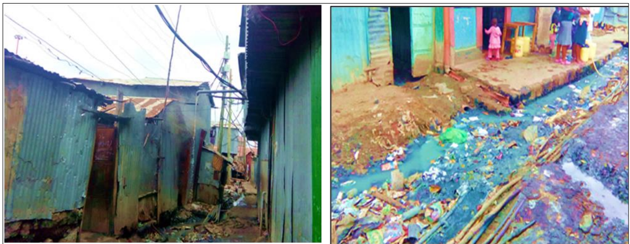
Figure 4.10: Water pipes running in unsanitary conditions in Section 48 and Moto Moto Villages
