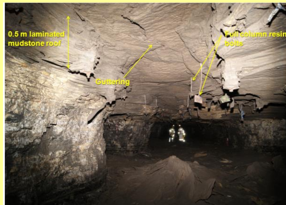
Figure 5-15 Picture showing a Multiple splits guttering at Kenako shaft resulting from a progressive slabbing of the laminated roof. Note that the bolts are still in place and do not seem to have been bent
