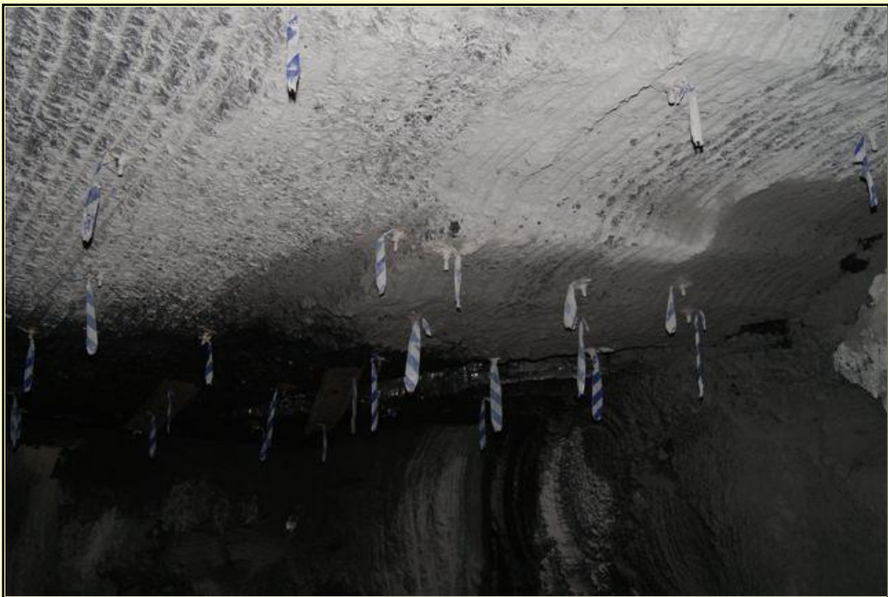
Figure 5-43 Picture showing the dyke visited at Boshmans and the presence of dripping water in the roof (X-Strata Coal)
