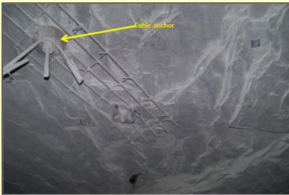
Figure 5-38 Picture illustrating the used of cable anchor in addition to roof bolts and metal straps
