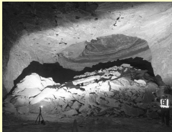
Figure 3-4 Large oval-shaped fall into the weaker overlying strata in a limestone mine (Esterhuizen et al, 2008)
