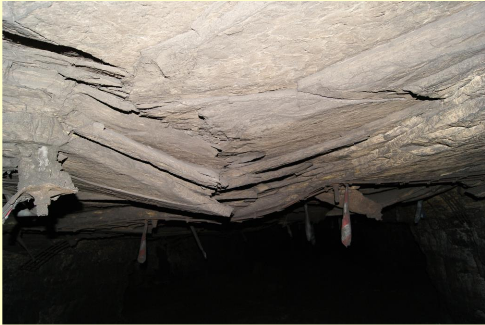
Figure 3-6 Picture showing a buckling roof at Kenako shaft in South Africa
