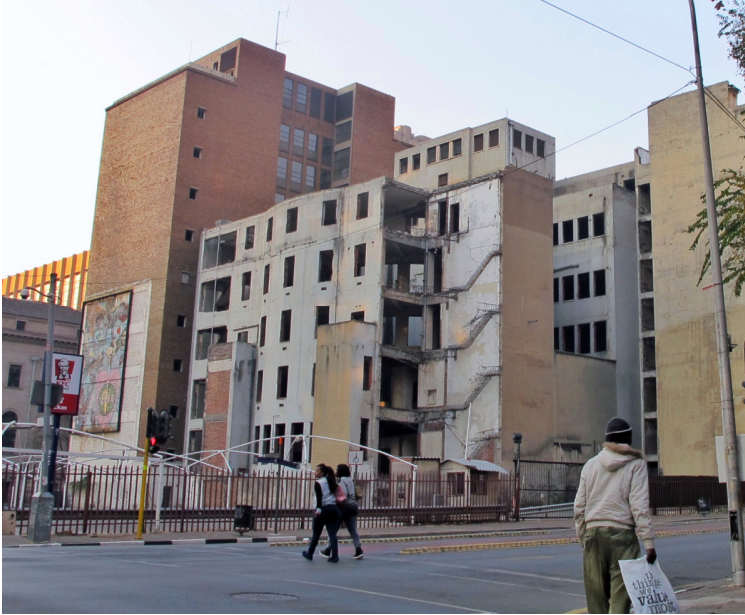
Figure 5: One of the many dilapidated buildings in the inner city, in contrast to the image below... (author's photograph).
