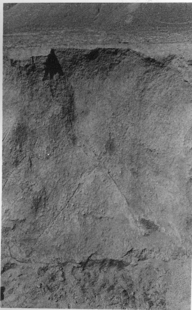
Looking east. Failure lines near centre. Note lines crossing.
