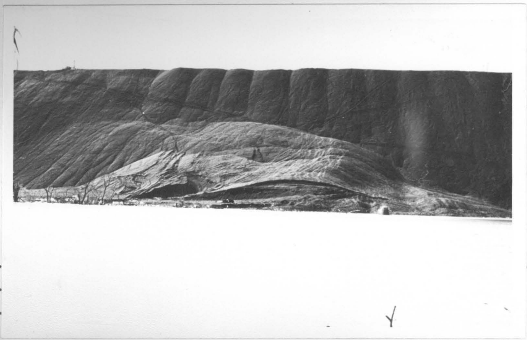
Figure 8.10 Failure of Sache's Dam East. The photographs show the secondary transverse failure lines very clearly. In the upper photograph at the top left-hand side of the failure note the horizontal ridges due to the primary failure. The bottom photograph (taken before Sache's Dam West was emptied) shows the infilling above the failure zone.
