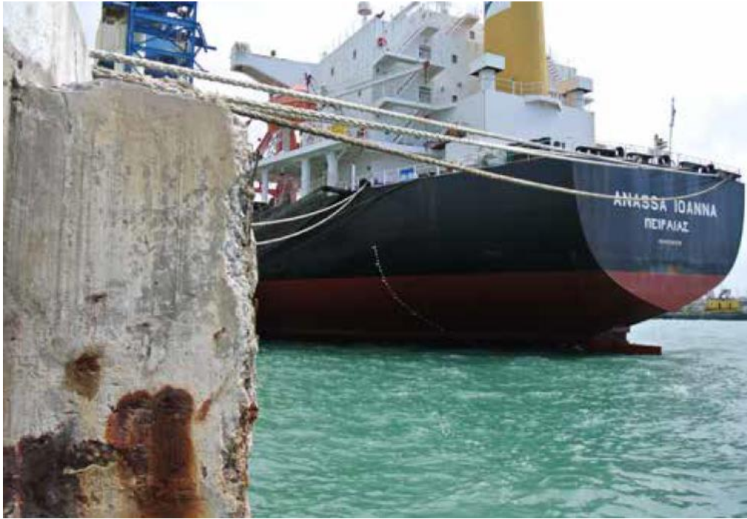
Figure 1.3: Chloride attack in concrete, (Source: Sika – Refurbishment Protective Coatings for Concrete)
