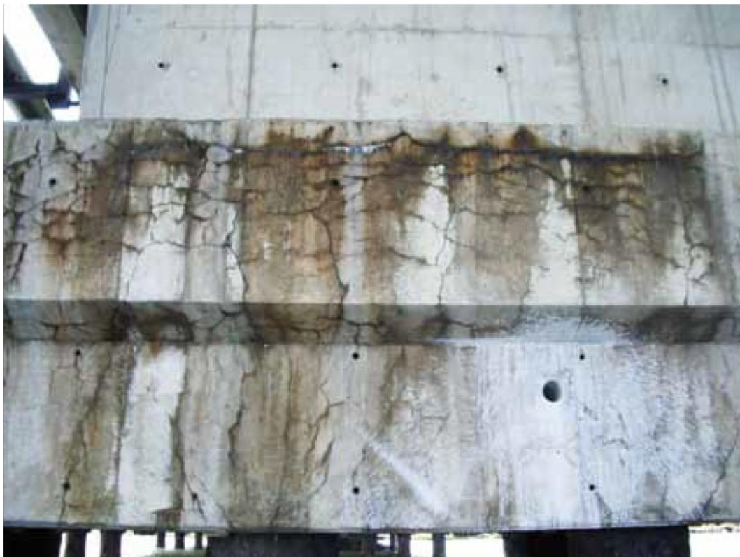
Figure 1.4: Alkali-silica reaction in concrete, (Source: Mapei – The Deterioration of Concrete)
