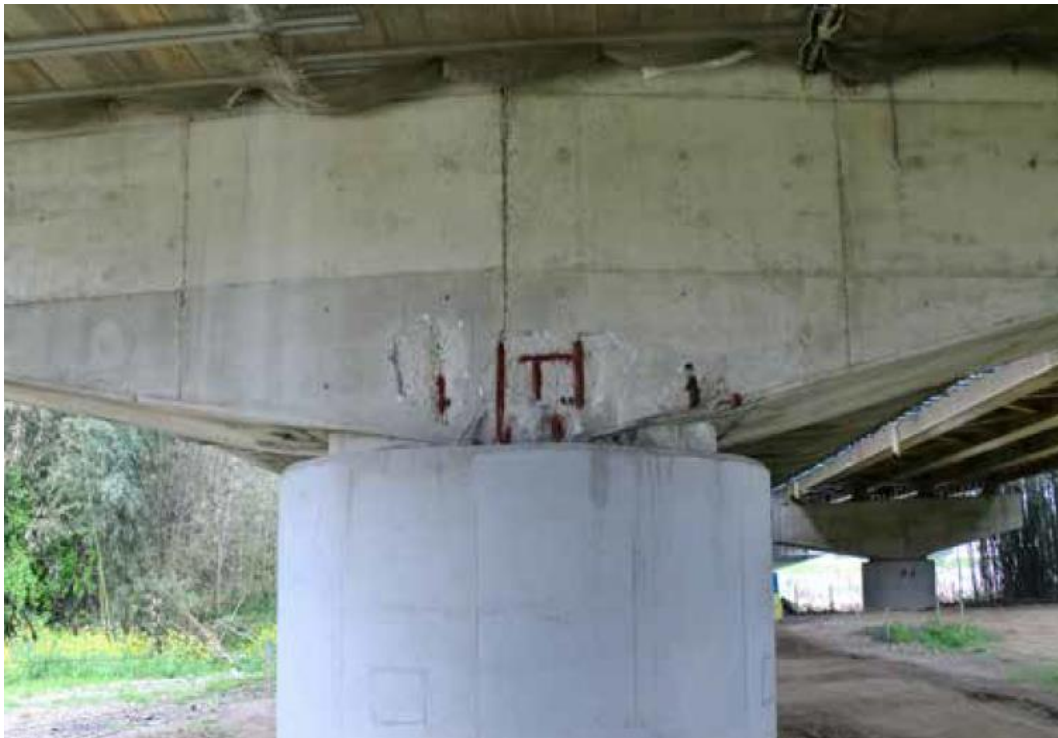
Figure 1.2: Carbonation induced corrosion, (Source: Sika – Refurbishment Protective Coatings for Concrete)
