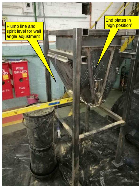
Figure 3-3 'High position' installation, indicating setup angle measurements
