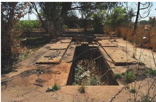
Foundations for two parallel mounted boilers
