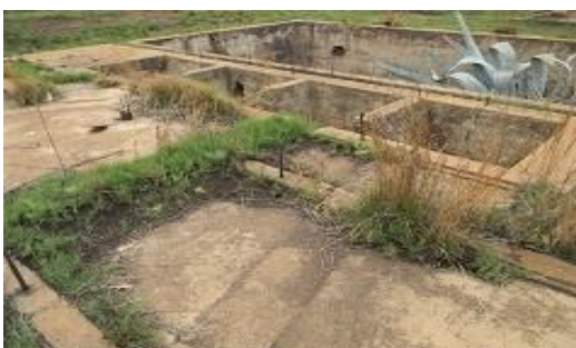
Various collection troughs beyond the MS flotation plant
