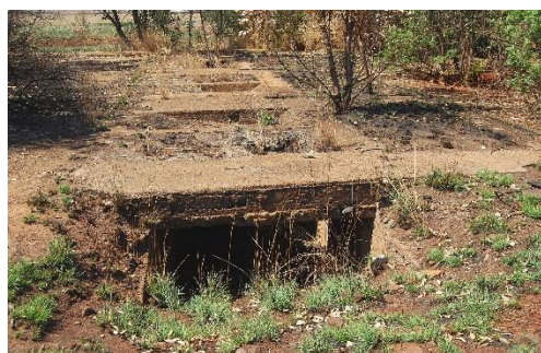
Figure 49. Ash chutes to lower railcar line used to carry ash to the dump.
