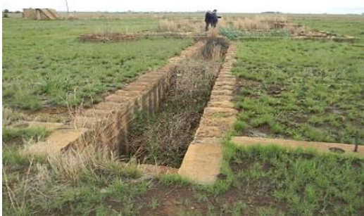
Close up of 1m deep trough between classifiers flotation and MS plant
