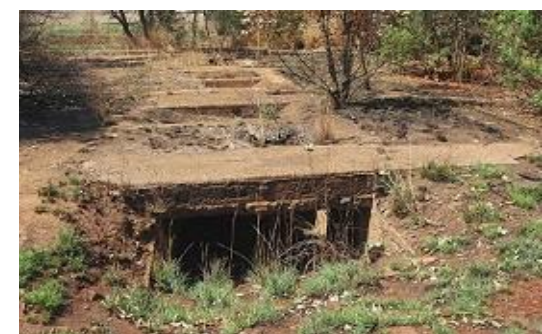
Ash discharge plates and coco pan tunnel underneath
