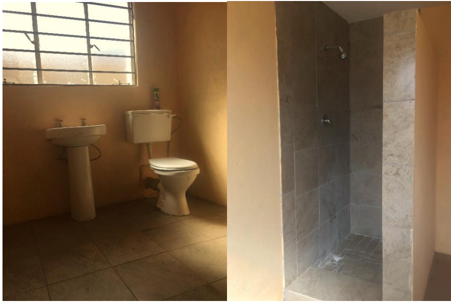
Figure 4.12: Shared toilet and shower facilities which are provided by L1 at her establishment in Lehae. Source: Mathibela, 2019.
