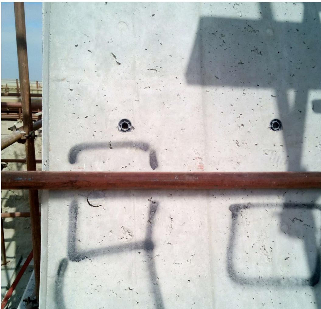
Figure 3-20 - Excessive blowholes on bridge abutment
