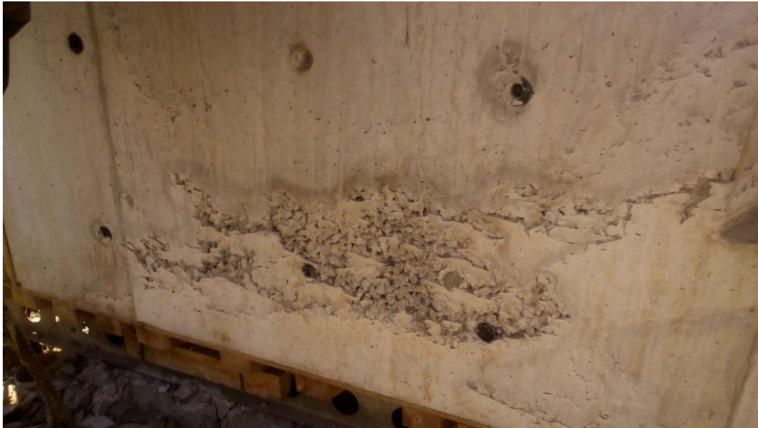
Figure 3-19 - Honeycomb on bridge deck diaphragm
