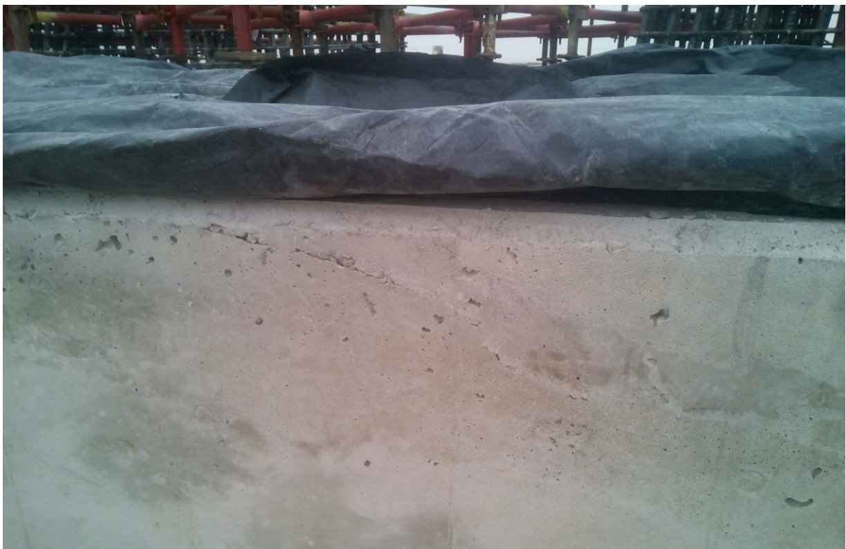
Figure 3-17 - Abutment footing showing inadequate vibration and cold joint
