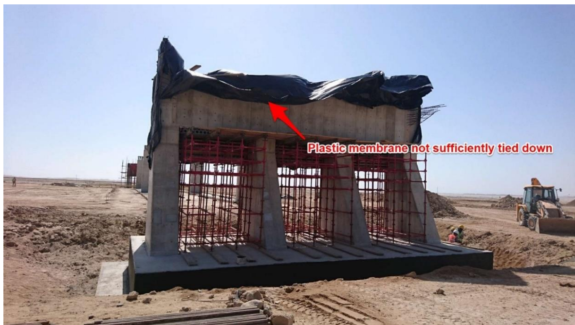
Figure 3-18 - Inefficient curing with impermeable membrane
