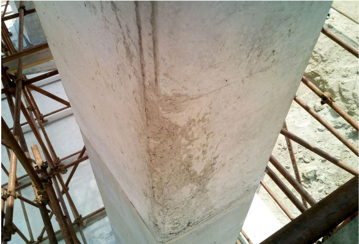
Figure 3-16 - Bleeding on bridge pier
