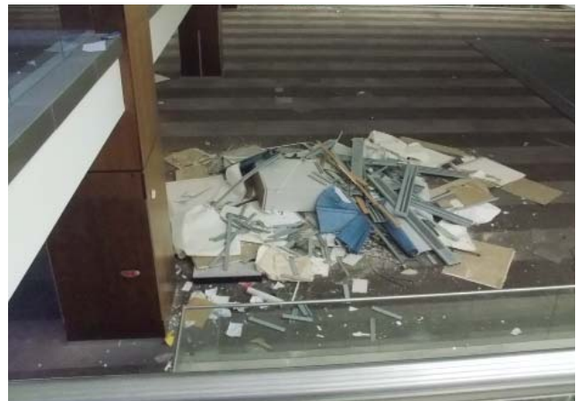
Fig 1.2: [Photograph by Author] Piled up construction waste on Site “Y”, which is the construction of a large low rise office block in Rosebank, Gauteng.
