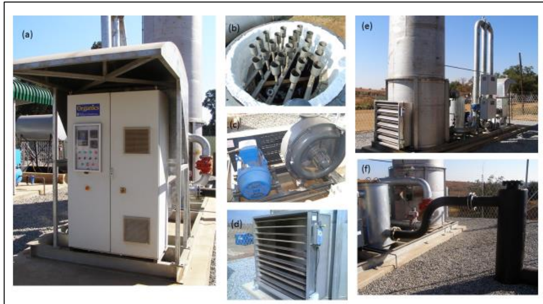
Figure 2.18: (a) Gas Delivery Unit (GDU) within the flare compound, (b) burners, (c) blower, (d) louvers, (e) flare and (f) LFG inlet feeding gas to the flare.
