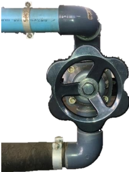
Figure 3-3- Discharge control valve
