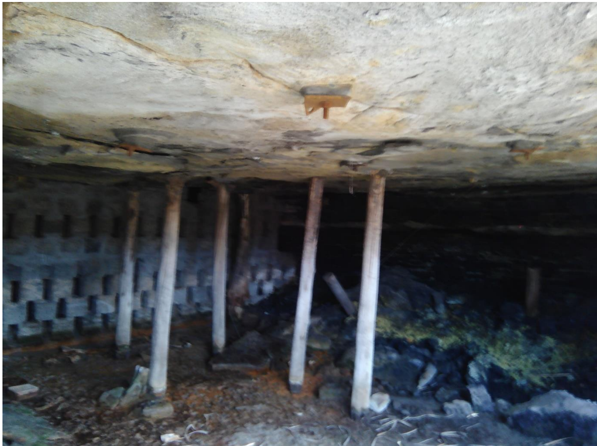
Figure 6.6. A mined-out opening that was accessed and had dimensions of 2 m thickness (stope width) and 4 m wide as was measured with a laser rule when accessed. Of interest is the single line brick wall built to offer roof support and keep illegal miners out.
