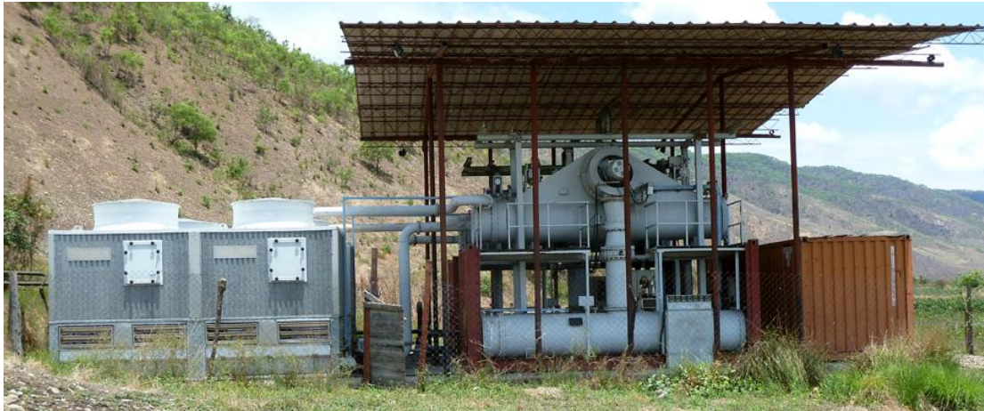
Figure 1.4. Pilot geothermal plant at Kapisya (courtesy of Kalahari GeoEnergy).
