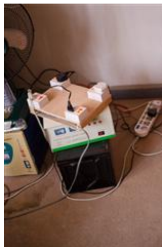
Inverter with batteries powering printer, fan, and other appliances. ( see larger )
