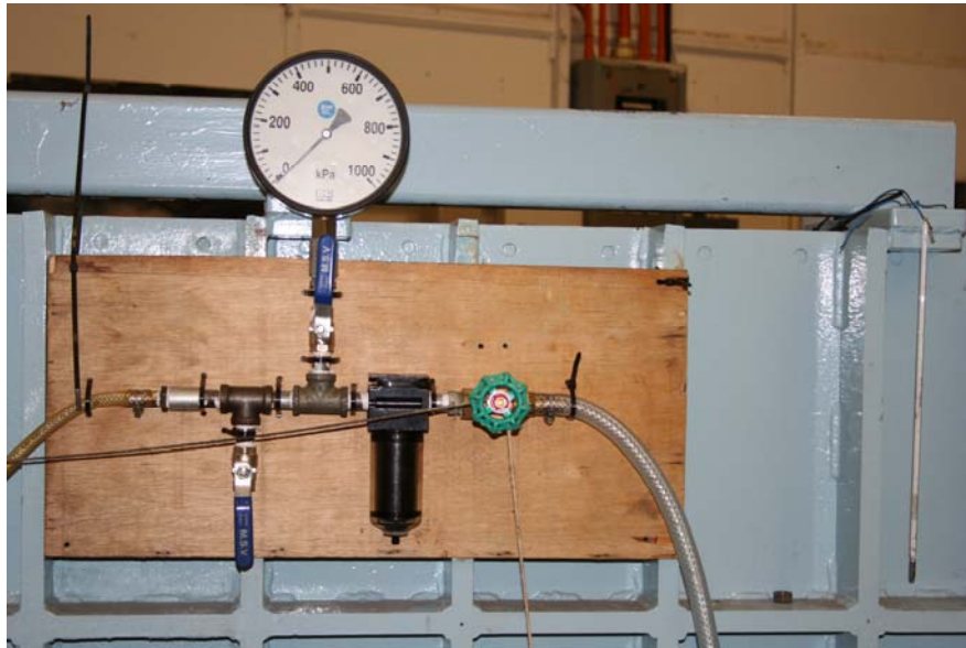
Figure 22: The control panel
