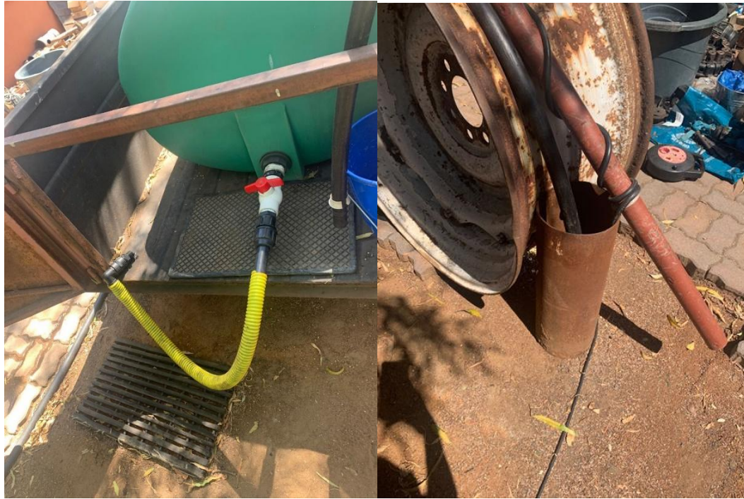
Figure 9: A picture shown depicts a borehole used for domestic supply with a storage tank.
