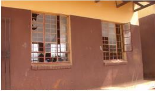
Image 1: Ithemba School's broken windows
