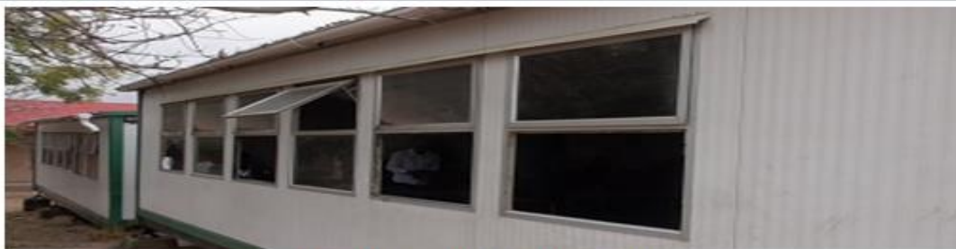
Image 1: Siyathuthuka's broken windows
