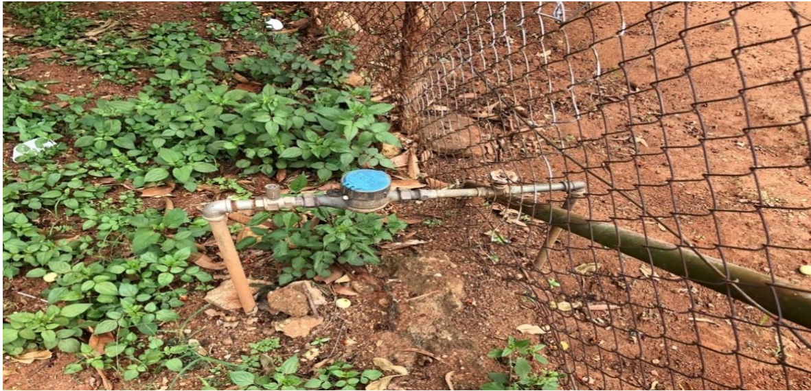
Figure 10: A water pipe connected into one of the units in Pusela 6
