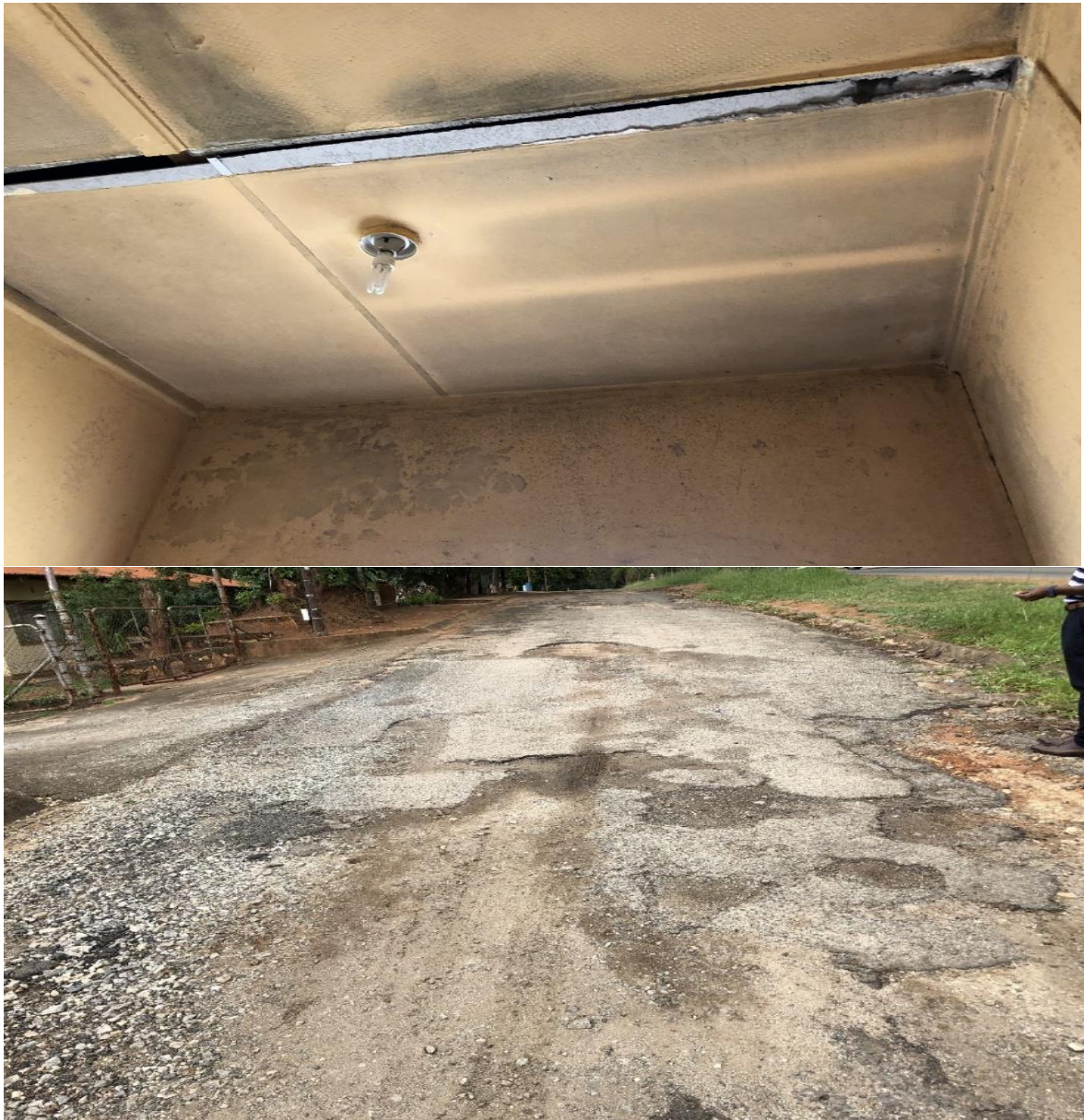
Figure 12: Pictures of public rental housing units in Pusela 6 showing the dilapidated ceiling and roads with potholes
