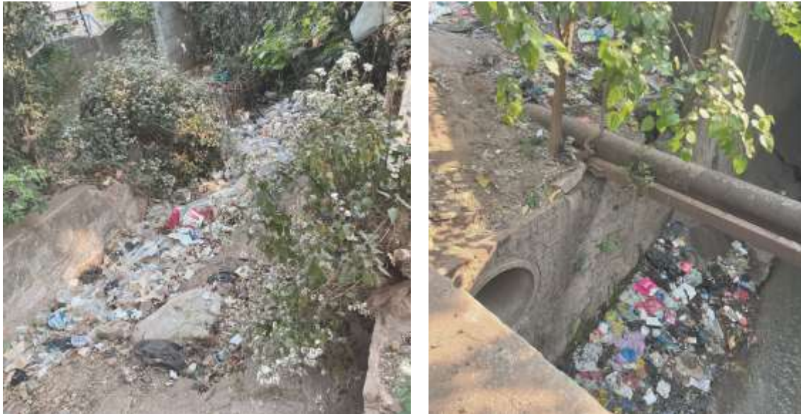
Figure 133: Existing stormwater runoff channels blocked by litter and alien vegetation (Photos by author)
