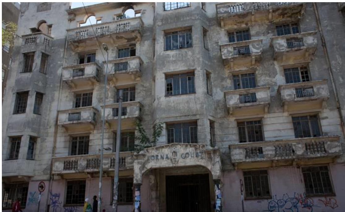
Figure 3.3: (above) Conditions of the Inner City – Image depicting the conditions of some of the buildings in the Inner City
