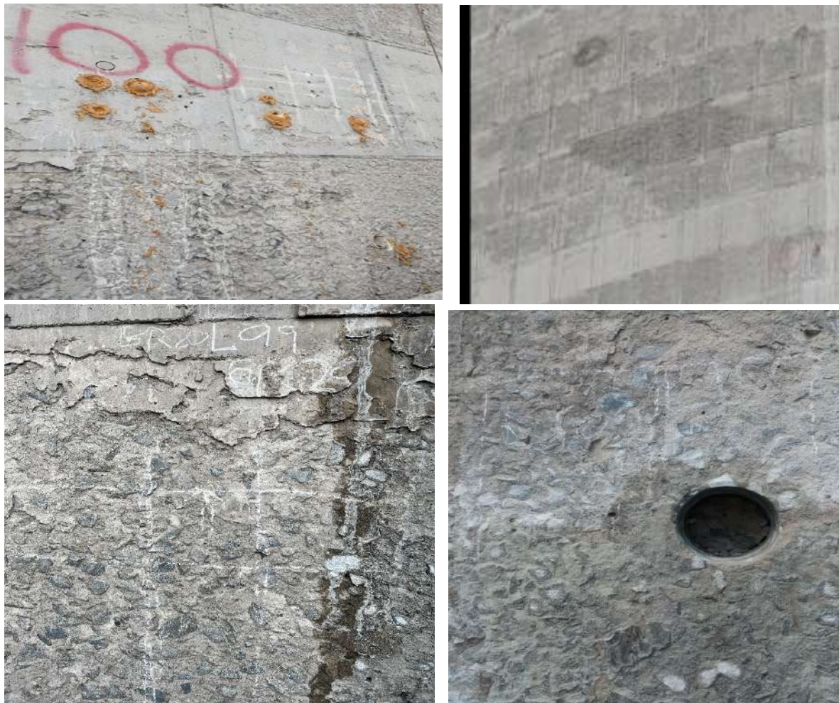
Figure 4-2: Varying concrete conditions at different locations of the tower
