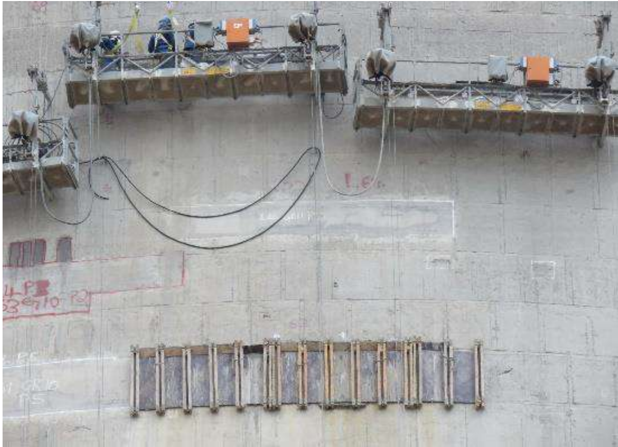
Figure 3-7: TSPs being supported by their associated guy ropes.
