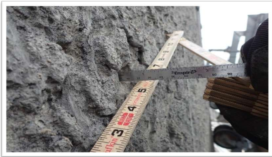
Figure 4-1: Exposed aggregate due to erosion of cement paste (Gries et al, 2022)
