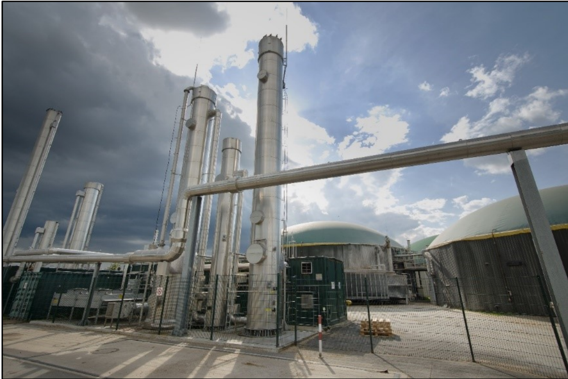
Figure 2.5: Modern biogas plant (Shutterstock Images, 2018)
