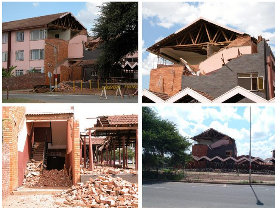
Figure 2.14 Damage to the Bel-Eaton court building during M_L 5.3 seismic event in Stilfontein area, source: van der Merwe, (2013)
