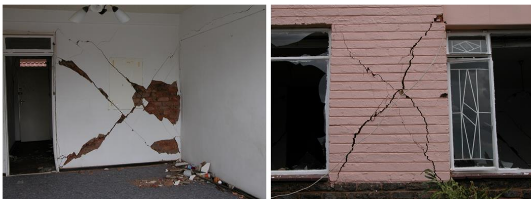
Figure 2.15 Damage to the masonry building during M_L 5.3 seismic event in Stilfontein area, source: van der Merwe, (2013)
