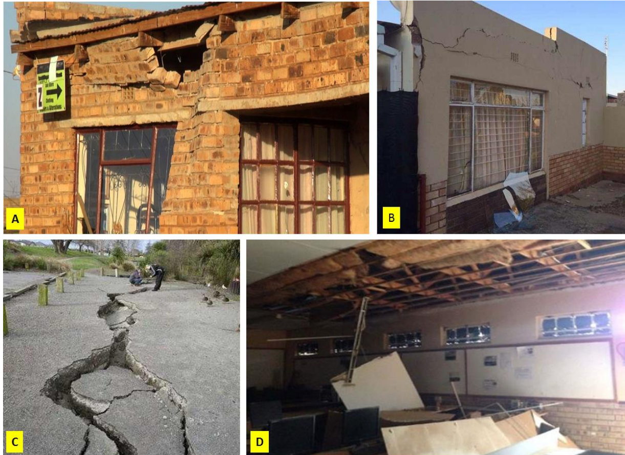
Figure 2.16 Damage due to M_L 5.3, Orkney seismic event on 5 August 2014. A; pointed masonry building, B; plastered masonry building, Vervaeck (2014) C; ground displacements, D; ceiling, Vervaeck (2014)
