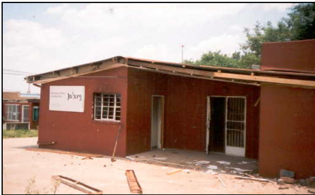
Photo 6.4. Burnt City of Johannesburg offices in Diepsloot
