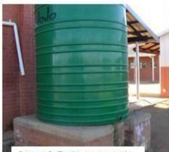
Image 3: Broken water tank
