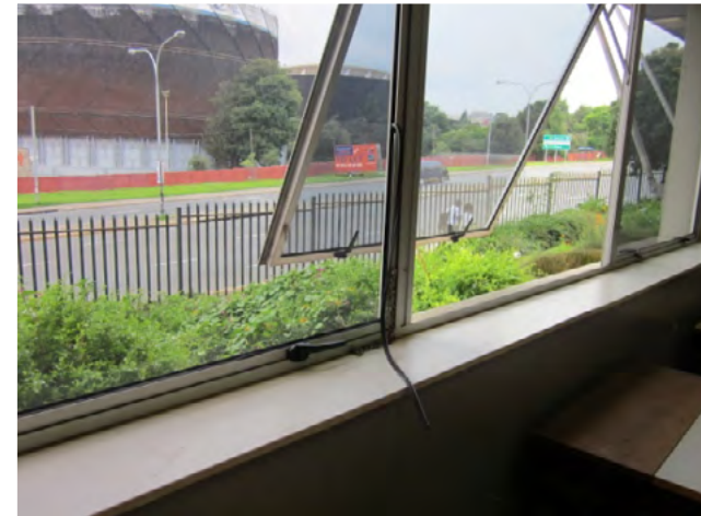
Figure 70: Studios that adjoin the north east-facing exterior façade receives ample natural light, but suffers from noise pollution and overheating in the afternoon. (Author, 07.02.2012)
