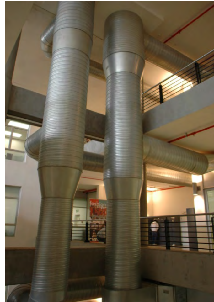
Figure 73: Exposed and oversized ventilation ducts cause noise pollution, UA (Author, 14.06.2009)
