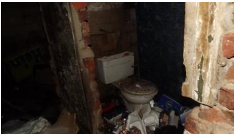
Figure 16 Broken toilet that is collecting waste
