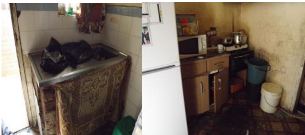
Figure 8 Blocked kitchen sink and cooking area
