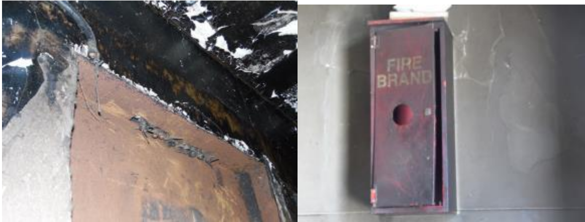
Figure 10 Transformer and broken fire extinguisher
