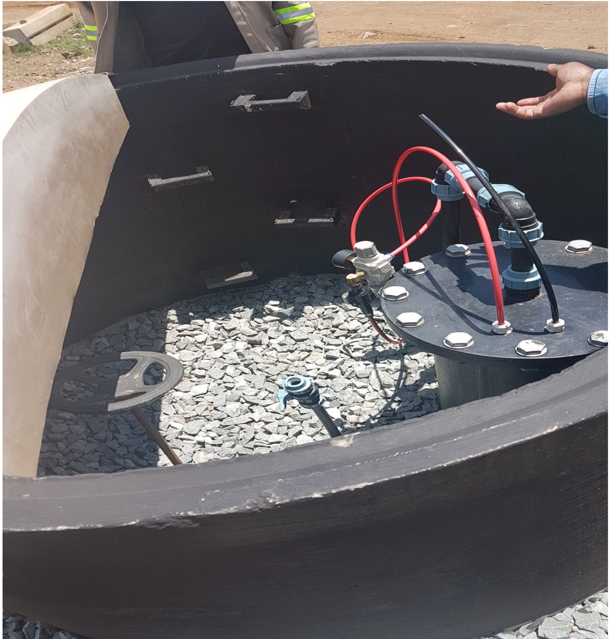
The above picture shows a landfill gas project in the city of Johannesburg
