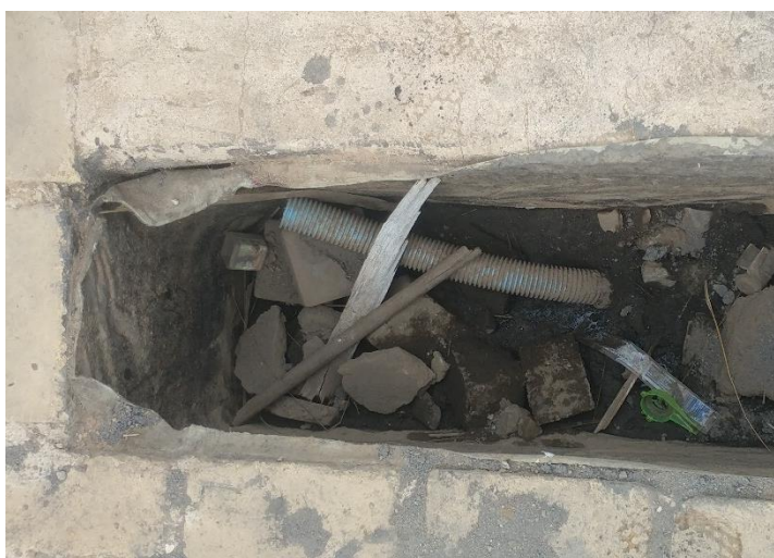
Figure 22: Outlet drain of constructed wetland 1 showing the blue flexible 'pool pipe' that connects the internal drain in the constructed wetland to the external drain. (Coordinates: 26°05'16.8"S 28°06'25.3"E)
