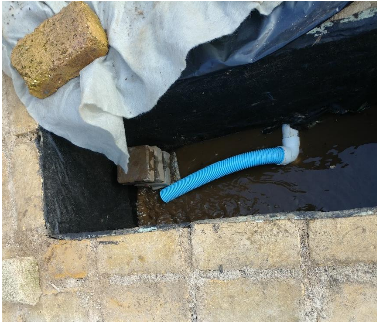
Figure 19: Exiting drain system of constructed wetland showing water flowing through flexible drainage hose
