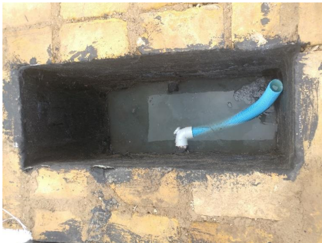
Figure 24: Outlet drain of constructed wetland 2. The blue flexible 'pool pipe' connects the internal drain in the wetland to the external drain which drain into an informal trench that leads to the Jukskei River. (Coordinates: 26°05'16.1"S 28°06'26.1"E)
