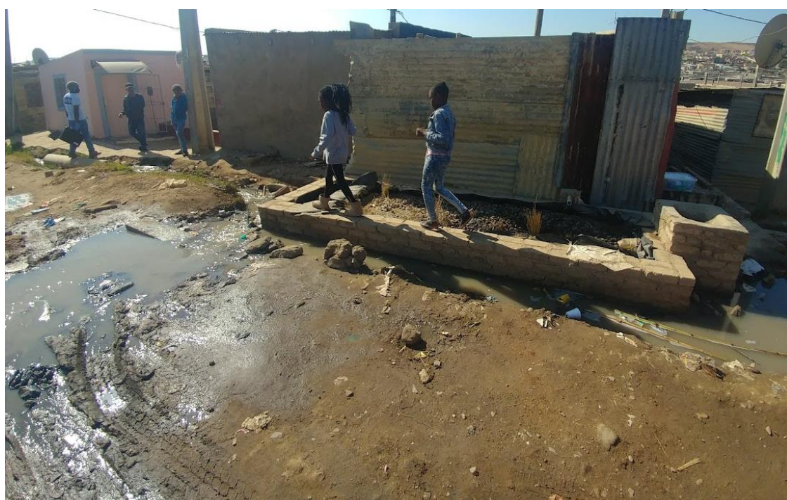
Figure 66: View of Constructed Wetland 1 on the 29th of July 2020 showing leaking sewage flowing adjacent to the retaining wall at a relatively high level. Two young girls are using one of the retaining walls as a bridge to avoid the leaking sewage.
