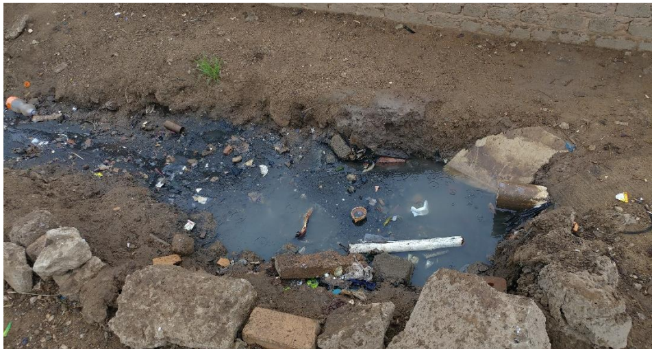
Figure 7: A typical shallow informal trench in Silvertown, Alexandra that links wastewater from communal tap (flowing into the trench via the PVC pipe on the right) to the Jukskei River
