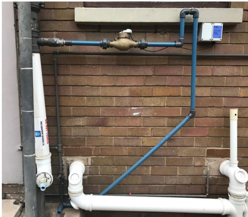
Figure 3. 18: Configuration of flow meter device on the Green Roof Pilot Project
