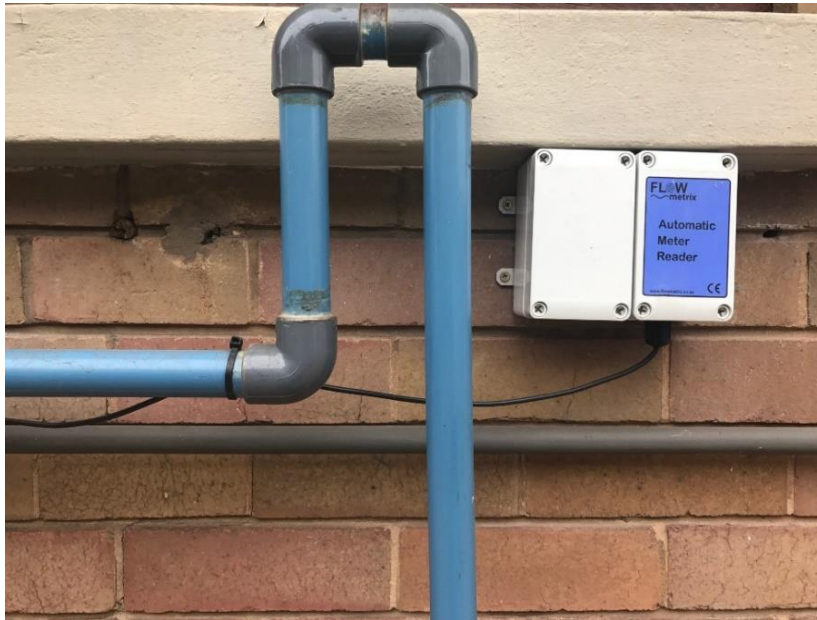
Figure 3. 19: Flow meter system used in the Green Roof Pilot Project
