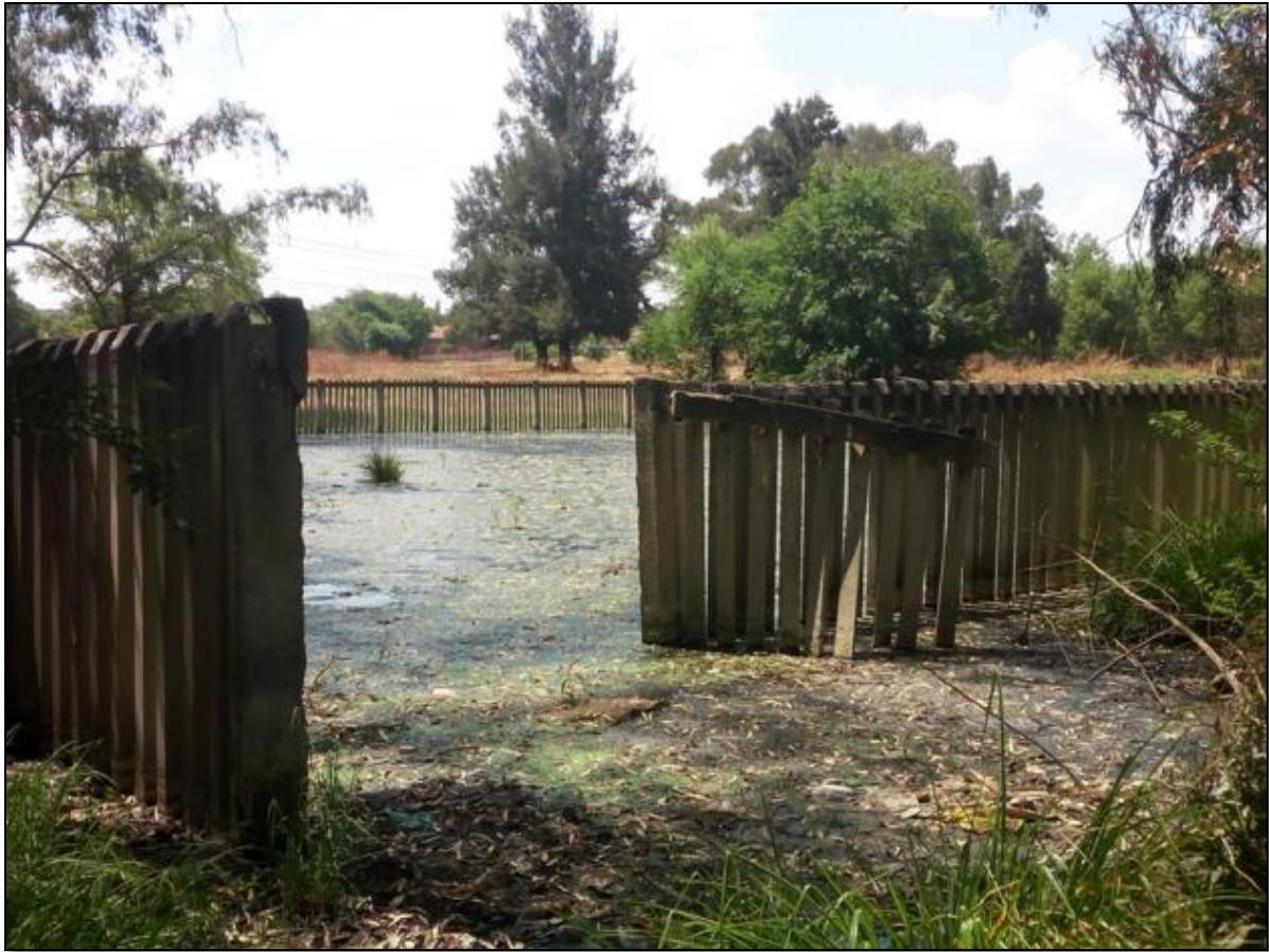
Photo 4.3: Overflowing emergency dam at pump station 8 (source: author's photograph, 18 October, 2019).
