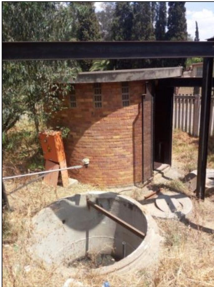
Photo 4.1: Dilapidated infrastructure at pump station 8 (source: author's photograph, 18 October, 2019)
