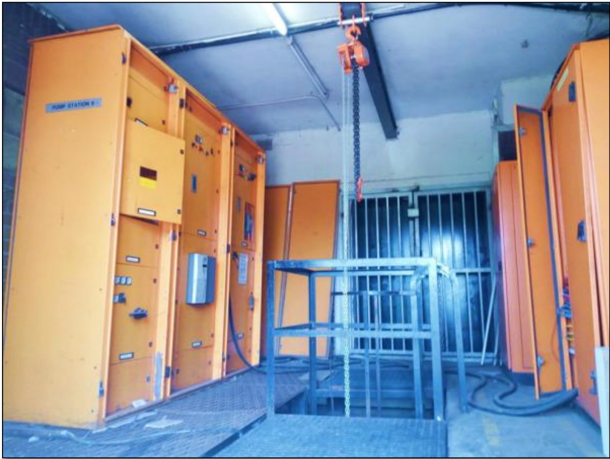
Photo 4.2: Unmaintained equipment inside pump station 8 (source: author's photograph, 18 October, 2019).
